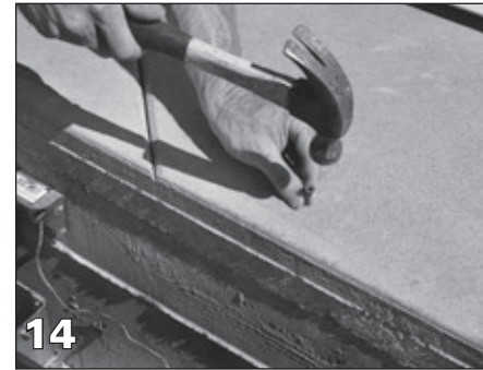
14 Remove the lid and hammer the plastic anchors (A1706) into the holes.
